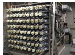
厨房排水処理設備 Kitchen wastewater treatment facility
